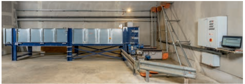
Dosing bunker with scraper floor for straw storage
